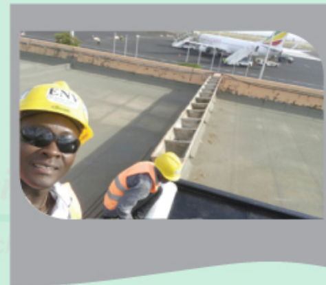
Waterproofing to Kilimanjaro International Airport (KIA) roofs – Rehabilitation project (Ref. HOLTAN E. A. Limited, P. O. Box 14131 Dar es Salaam and; BAM International bV., P. O. Box 78809, Dar es Salaam)
