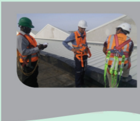
Waterproofing technical roofs for Julius Nyerere International Airport Terminal III (Ref. BAM International bV., P. O. Box 78809, Dar es Salaam)
